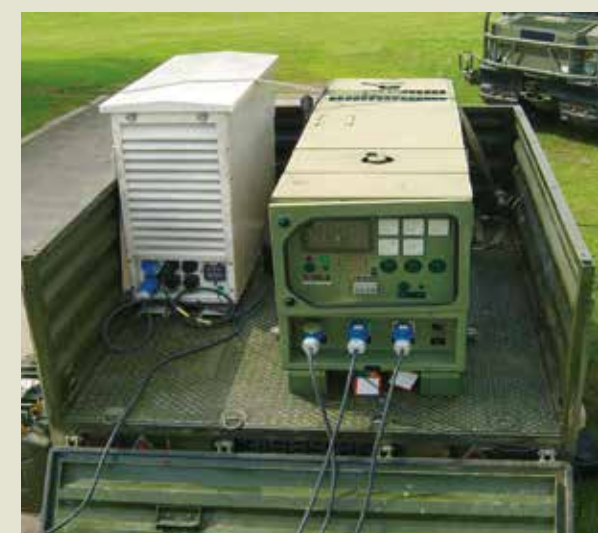
Fully self-contained generator with fuel tank, electrical cabinet. This generator is being used to power a SATCOM unit.
