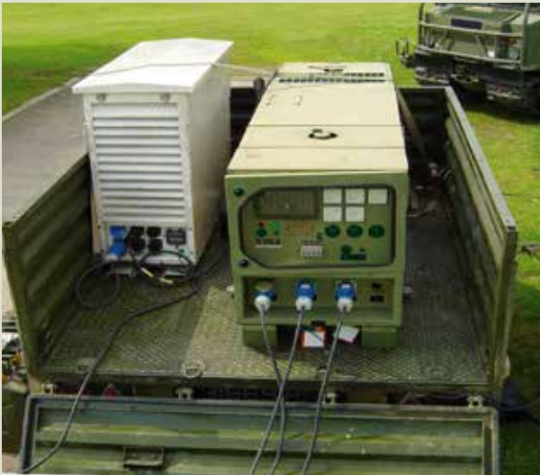
Fully self-contained generator with fuel tank, electrical cabinet. This generator is being used to power a SATCOM unit.
